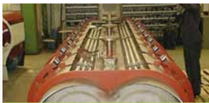
Jacket steam piping
