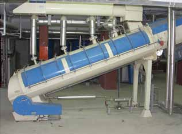
Super conditioner preparation stage on pellet mill
