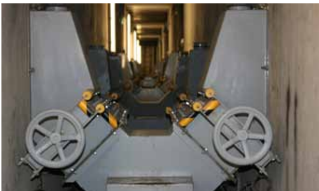
Valves under cells
