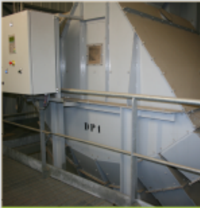
Swing spout distributor and control cabinet
