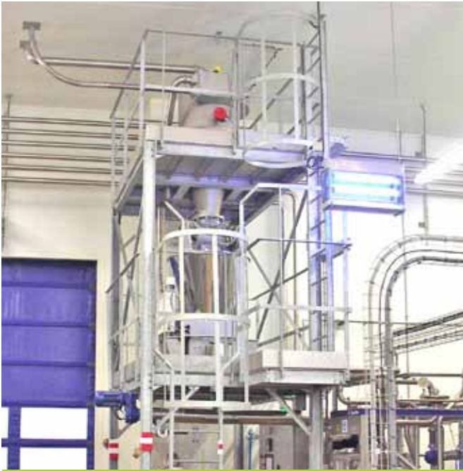
A pneumatic transfer supply by cyclone
