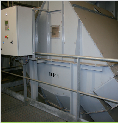
Swing spout distributor and control cabinet
