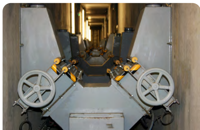
Valves under cells
