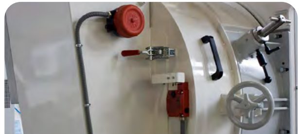
Safety device on electrical doors
