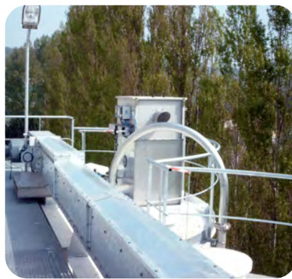
Pad filter for silo depressurization
